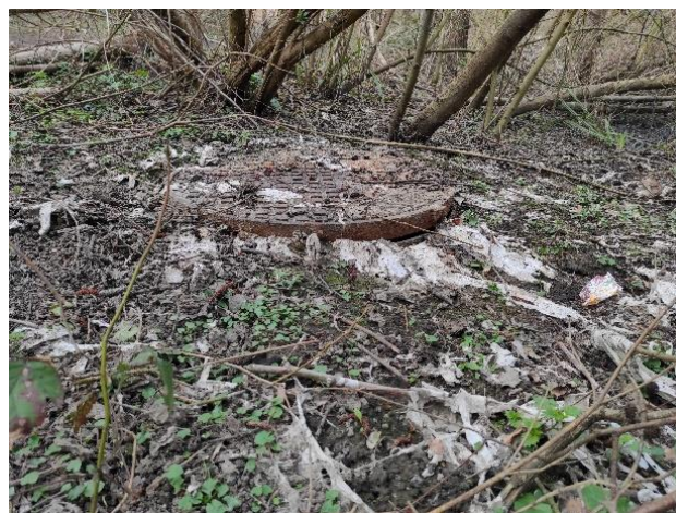
Overstroomde afvalwatercollector © CCN
